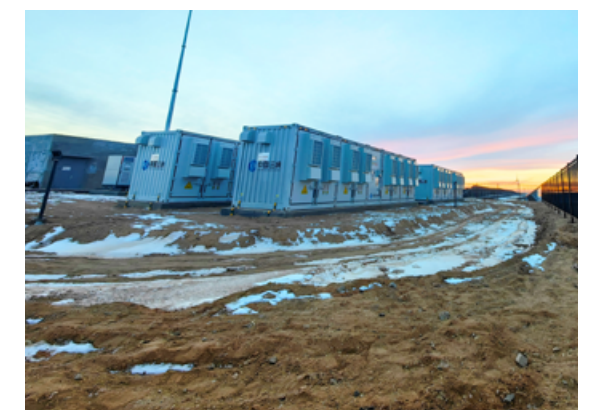
Mazongshan 50MW PV storage project
