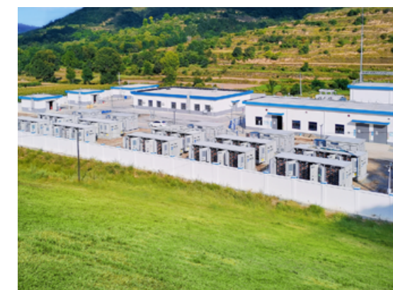
Qingshui Huangmen 100MW Agri-PV and Storage Integrated Power Station
